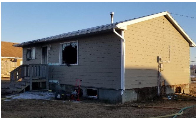
A structure fire, April 20, 2022
