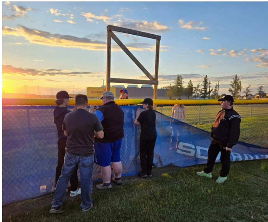
Members of the 15U Sox install the wind screen on the outfield fence of Diamond 2 in Lions Park
