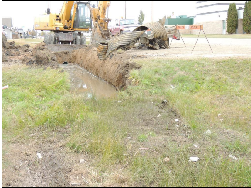
Figure 19: Removal of the existing storm pipe and installation of a new pipe on the approach road to the Alliance Church
